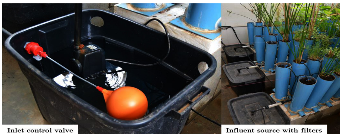
Figure 3. Flow inlet control and submersible pump and a depiction of the irrigation filters
