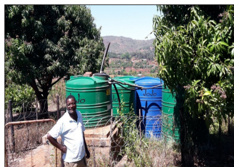
Figure 4. Storage tanks Mulangapuma 1
