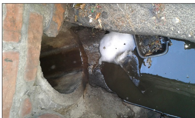
Figure 12. Carwash effluent discharging into Manhole 19MON
