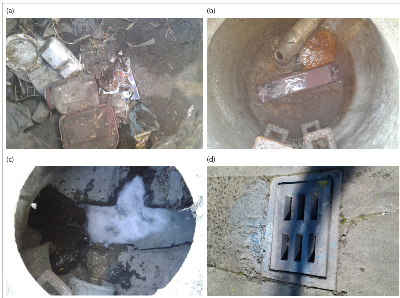
Figure 17. Photos of illegal discharges in manholes on Alternator Avenue: (a) Manhole 5ALT filled with stones; (b) Manhole 11ALT with pinkish discharge; (c) Manhole 7ALT with white soapy foam discharge; (d) stormwater inlet with stain
