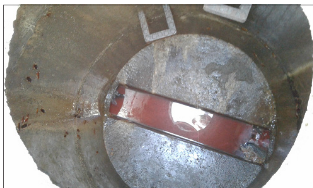
Figure 15. Photo of deep maroon colour discharge in Manhole 4FOU
