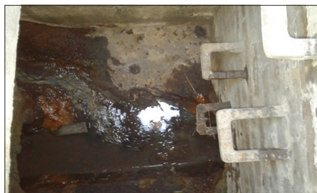
Figure 16. Photo of an illegal discharge in Manhole 17CHA
